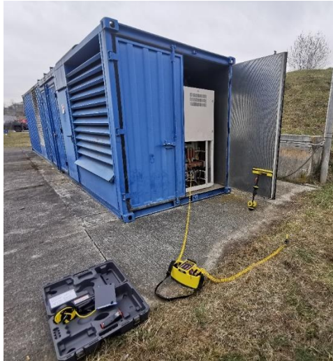
Fig. 6.1 Connecting the Ridgid SeekTech ST-510 line transmitter to the faulty cable
