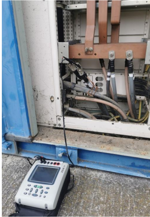
Fig. Error! No text of specified style in document..3 Connecting the Megger TDR2000/2R reflectometer to the faulty cable
